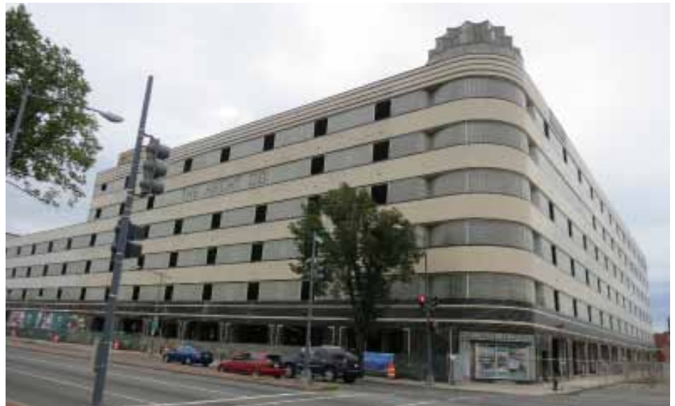
TOP: 1500 Massachusetts Avenue, SE. BOTTOM: Hecht Co. Warehouse, 1401 New York Avenue, NE under renovation (August 2014).
