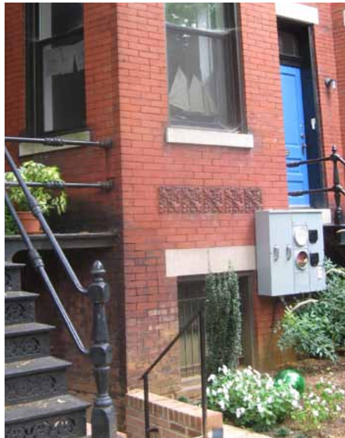
Home renovations and improvements have left many Hill front façades with large, unsightly electrical boxes.
