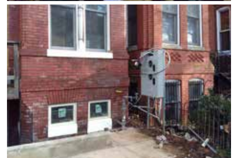
Non-compliant electrical meter boxes.
