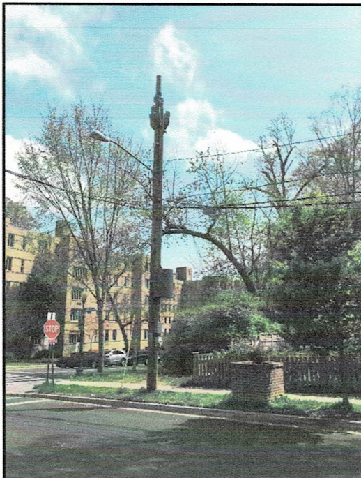
2900 block of Garfield St NW with Small Cell installation
