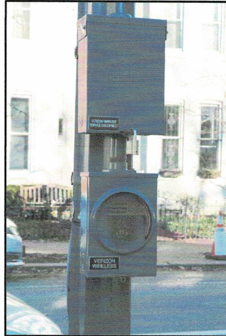
Close up of the meter and disconnect boxes
