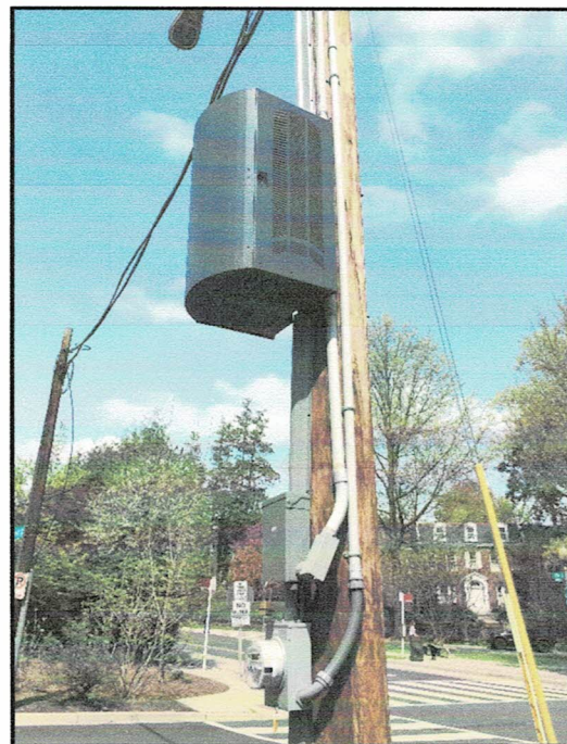
Close up of the cabinet, meter and disconnect box
